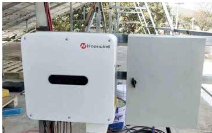
Residential PV Project in China
