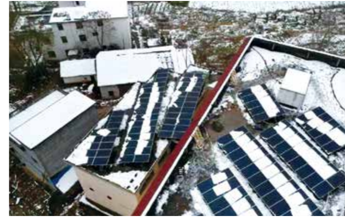
Solar Power Project in Jiangxi, China
