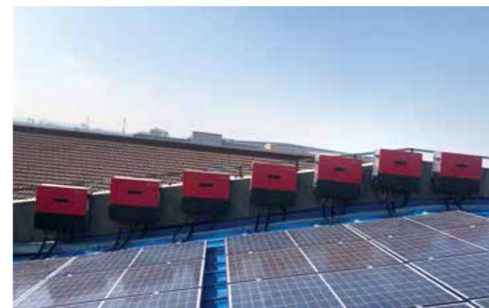
Rooftop PV Project in Jiangsu, China
