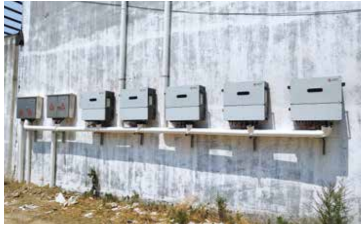
Rooftop PV Project in Shandong, China
