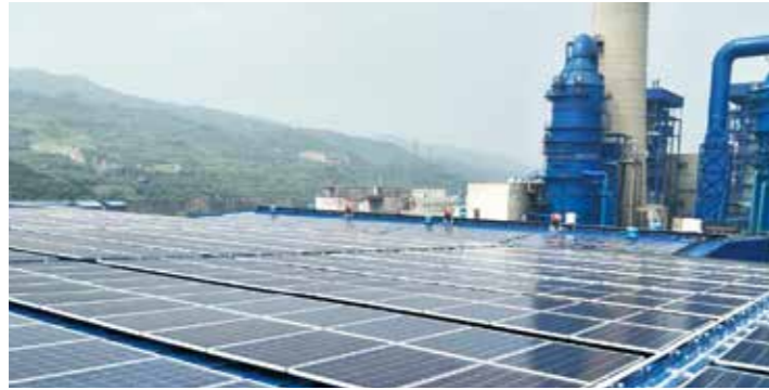
Operation of 50kW String Inverter
