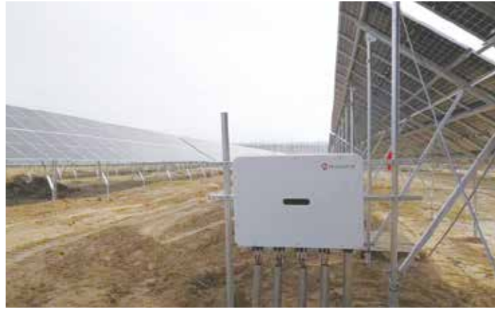
200MW hopeSunHV250KTL Utility Project in Ningxia, China
