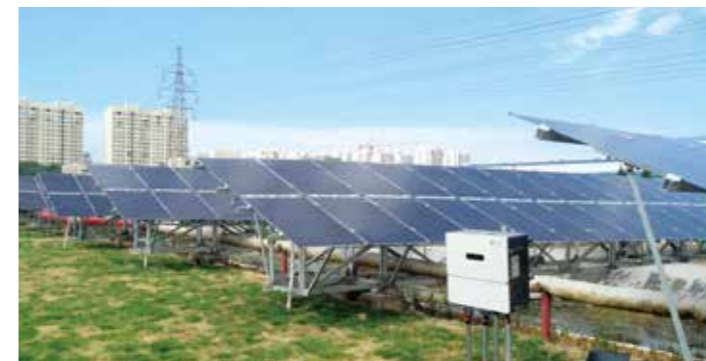
CNNC 2.8MW PV Project in Shandong, China
