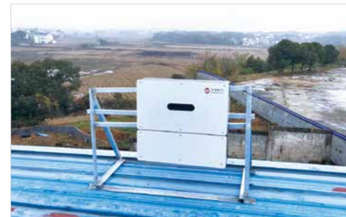
Rooftop PV Project in Hunan, China
