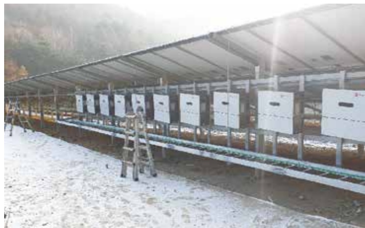
550kW Solar Plant in South Korea
