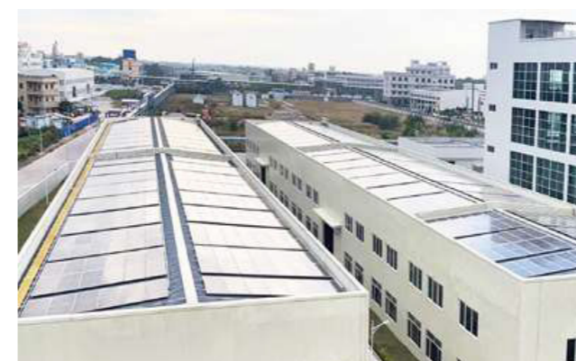
Baoying Rooftop Solar Power Station
