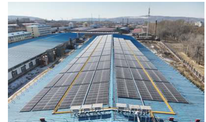
Muling Rooftop Solar Power Station
