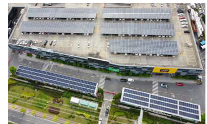
Our Choice Rooftop Solar Power Station
